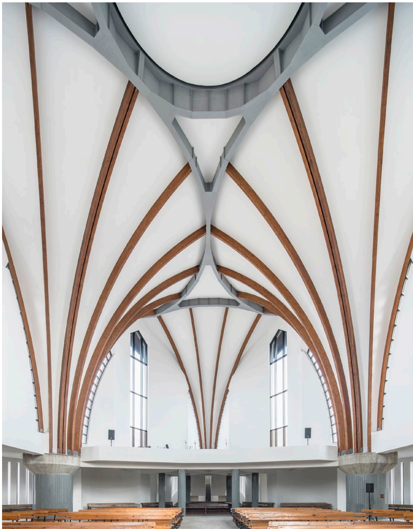
Progetto: Roman Catholic Parish, Toruń, Polonia Installatore: ProSystem Krzysztof Dziewulski / Controsoffitto: Rockfon® Mono® Acoustic
